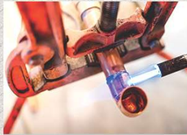
WATER PLUMBING SERVICES
