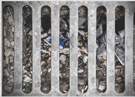
SEWER PLUMBING SERVICES
