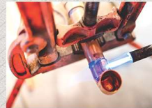
WATER PLUMBING SERVICES
